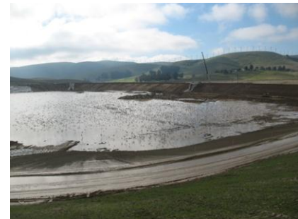
The 425-AF Dyer Reservoir under construction in January 2011 as part of the South Bay Aqueduct Enlargement Project.
