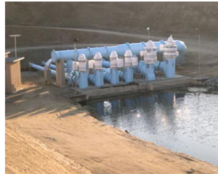
Groundwater banking facilities at Semitropic Water Storage District. (Source: http://www.semitropic.com/Facilities.htm )
