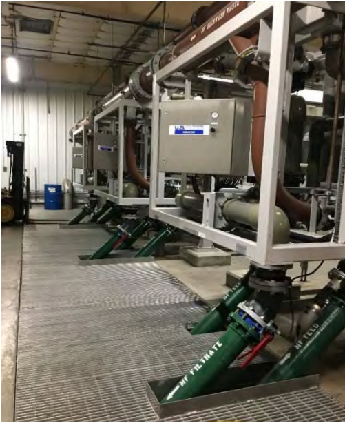
Figure 7.8 DSRSD Microfiltration (MF) Building
