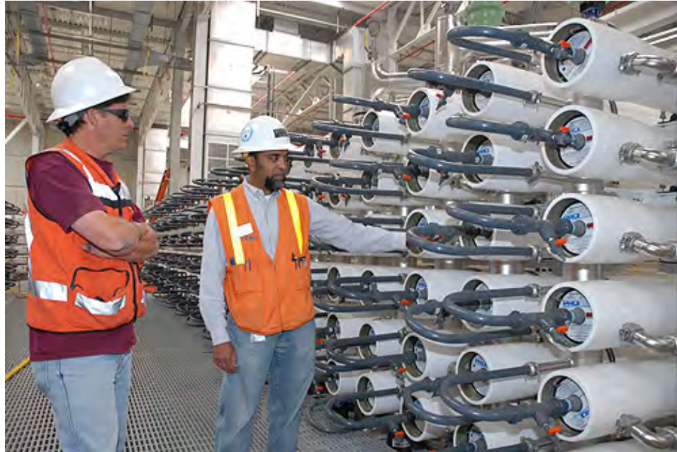
Figure 2.2 OCWD RO Membranes Used to Purify Reclaimed Water for Potable Reuse
