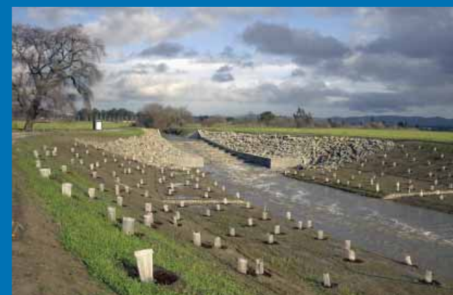
A Zone 7 restoration project along Arroyo las Positas near El Charro Road involves planting of native vegetation to keep the bank from eroding, as well as a fish ladder to help fish migrate upstream.
