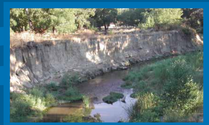
Bank erosion on Arroyo de la Laguna can cause bank instability and deposit sediment in the arroyo.
