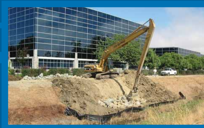
Zone 7 performs routine maintenance such as inspections, repairs, vegetation management, silt removal, pest control, and other activities that keep channels in smooth working order. Zone 7 also conducts emergency repairs and installs new channels as necessary.
