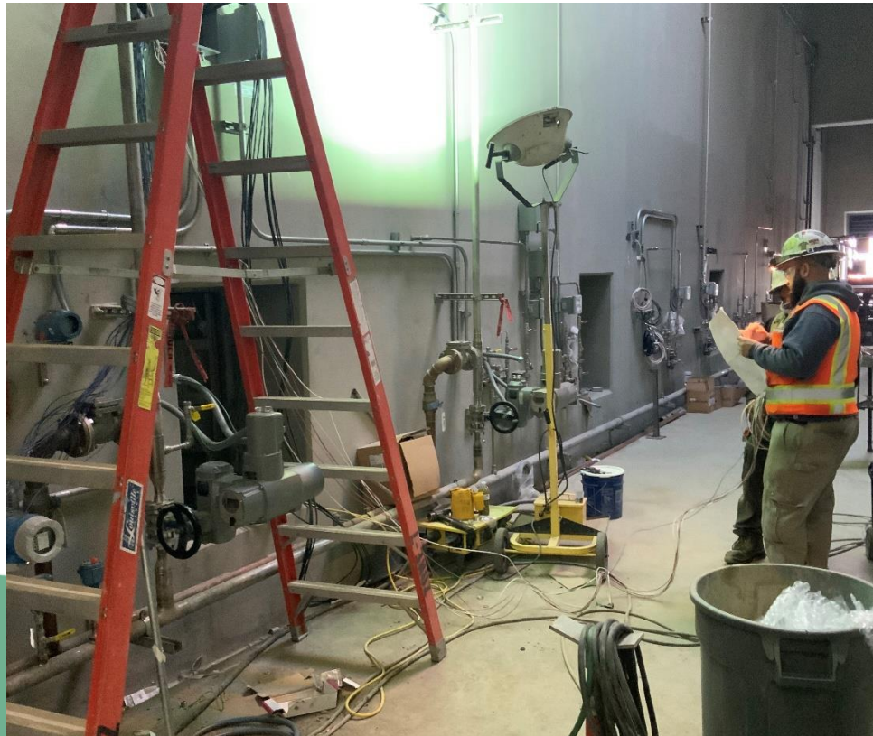
General View of Ozone Contactor Gallery – 12/1/21
