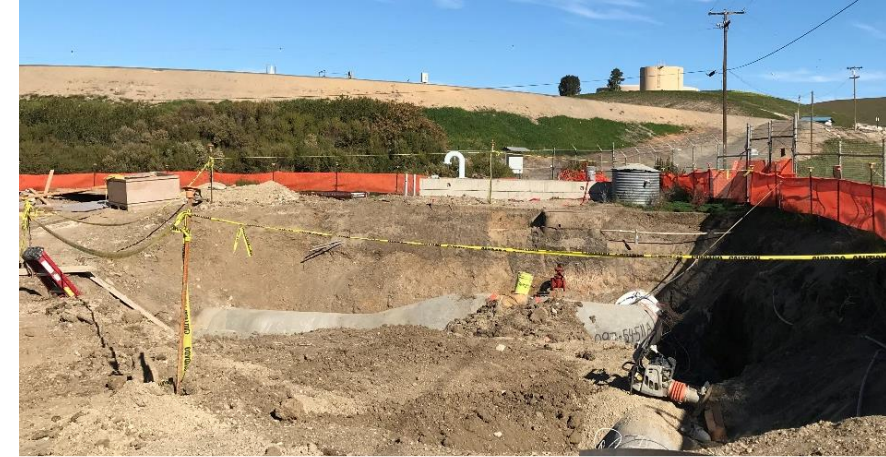
Inlet Piping & Ozonation Water Piping – 2/10/22
