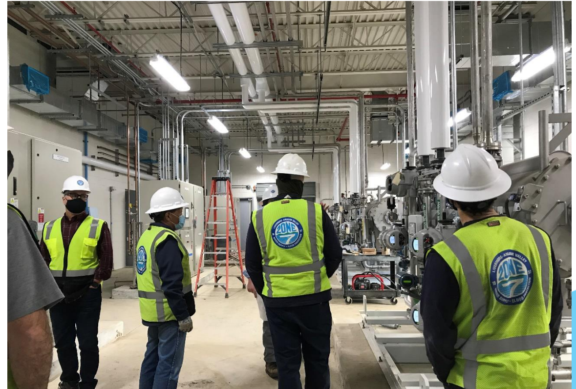
General View of Ozone Generation Building (with Lighting) – 1/19/22
