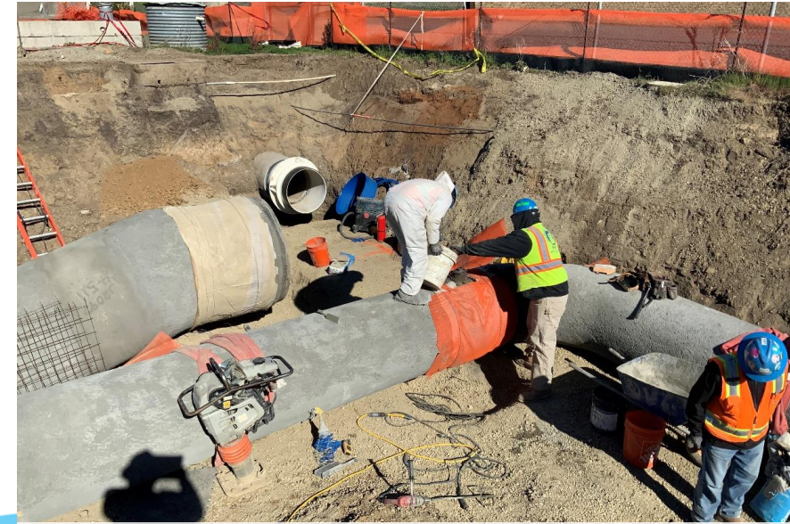
Inlet Piping & Ozonated Water Piping – 2/2/22
