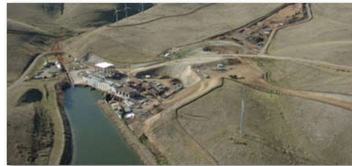
State Water Project's South Bay Aqueduct is being improved and enlarged to meet contractual capacity levels.
