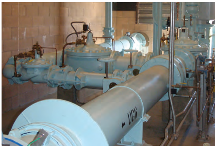
Two new Chain of Lakes wells went into operation in 2010.
