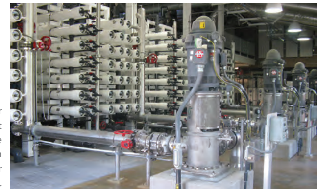
The Mocho Groundwater Demineralization Plant demineralized 2,400-acre feet (more than 782 million gallons) of groundwater in 2010.
