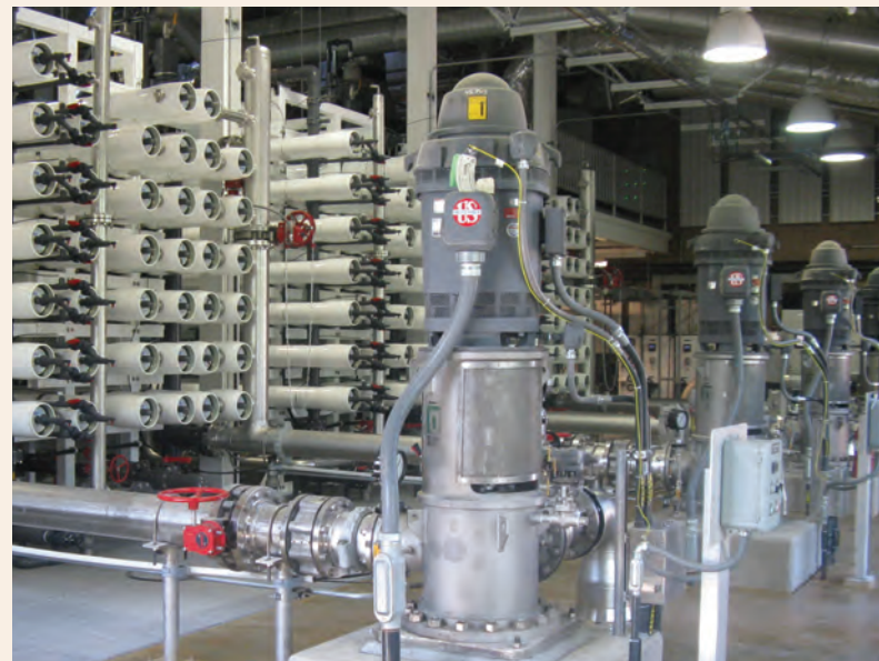
The Mocho Groundwater Demineralization Plant
