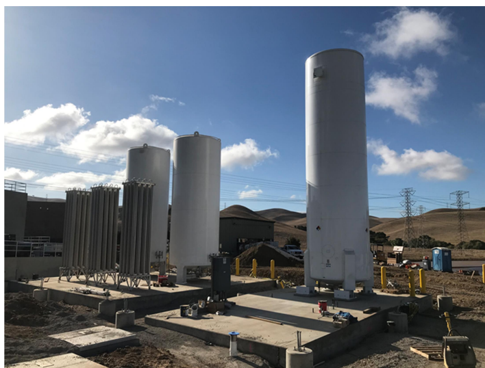
New liquid oxygen and carbon dioxide tanks at the DVWTP Ozone facility.
