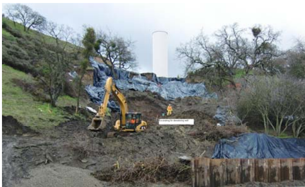
Damage to the Del Valle Branch Pipeline in December 2009
