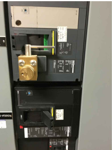
EXISTING 1000A BREAKER
