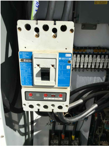
EXISTING 400A BREAKER
