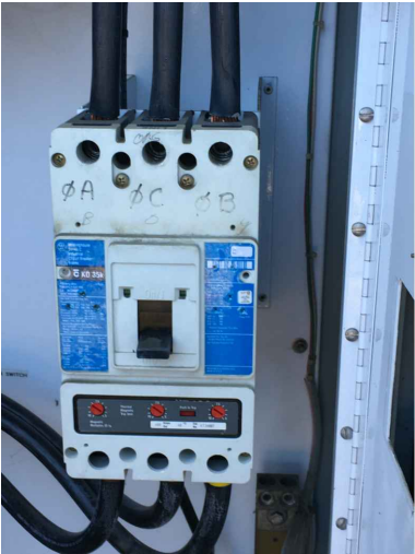
EXISTING 400A BREAKER
