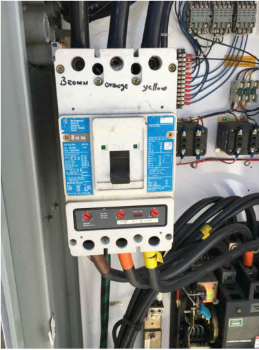
EXISTING 400A BREAKER
