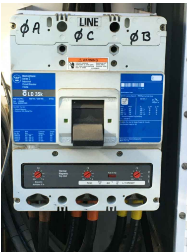
EXISTING 600A BREAKER
