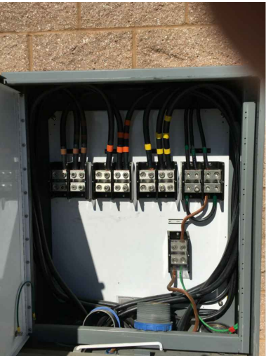
EXIST ELECTRICAL BOX
