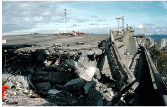
Collapsed Cypress viaduct
