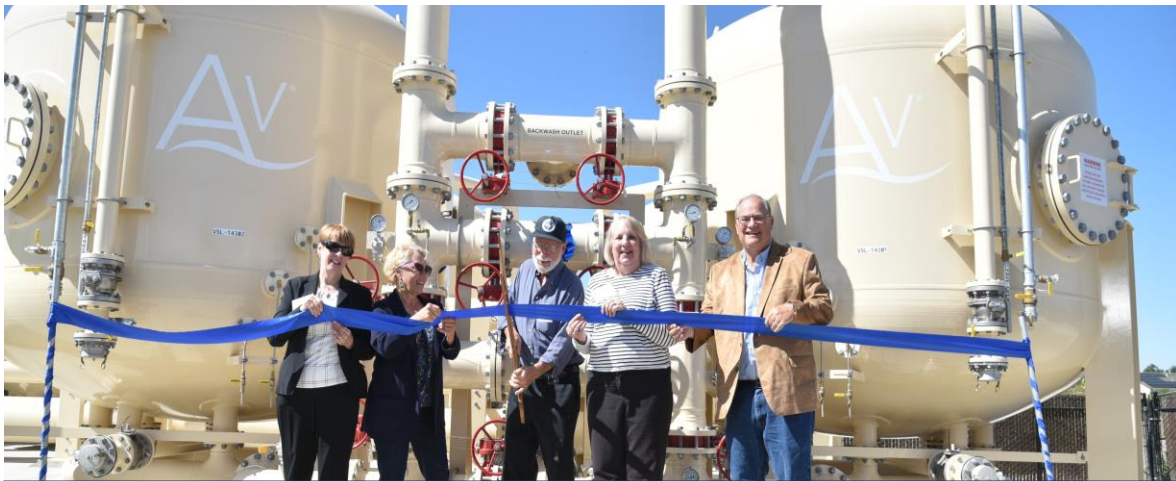
Stoneridge PFAS Treatment Facility
