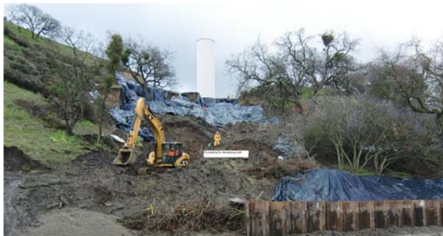
Damage to the Del Valle Branch Pipeline in December 2009
