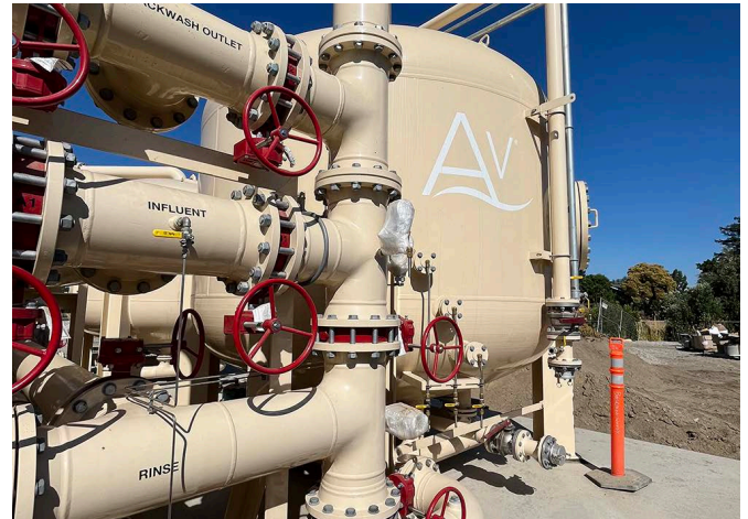
Ion Exchange PFAS Treatment System installed at the Stoneridge Well, the first of its kind in Northern California
